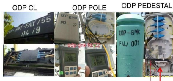
Figure 8. Optical Distribution Point
