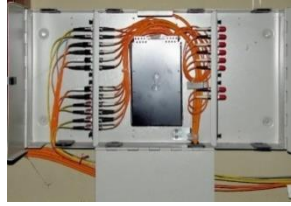
Figure 4. Optical Distribution Frame
