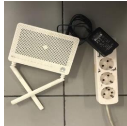
Figure 10. Optical Network Termination
