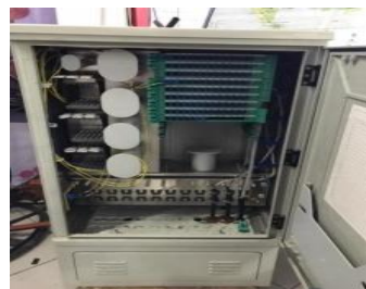
Figure 6. Optical Distribution Cabinet
