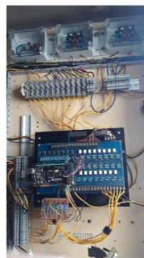
Figure 13. Unit ECC Unit in Electric Control Panel of Crane Ferrari178H1
